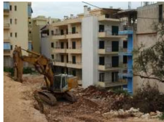
Fig. 8: Transforming of the Mediterranean vegetation by uninhibited construction activities.
